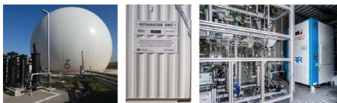
Methanation unit in EDAR (Sabadell)
